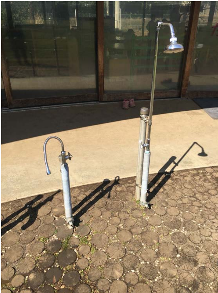
Left - Water taps in courtyard teach children how to control and turn on taps manually.
